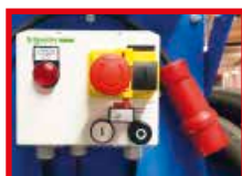
Single-phase electrical panel
