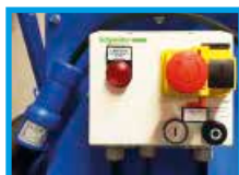
3-phase electrical panel
