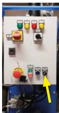
Start/Stop auxiliary pump for particle counter Fig.13
