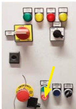
With electric indicator and particle counter Fig.18
