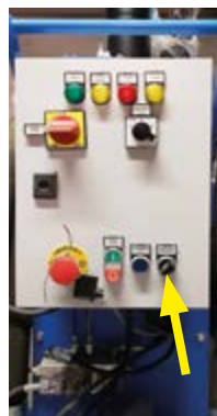
Start/Stop auxiliary pump for particle counter Fig.14
