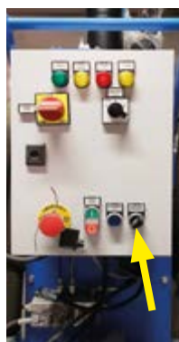
Start/Stop auxiliary pump for particle counter Fig.15
