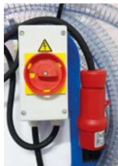
3-phase electrical panel
