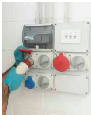
Electrical connection for the three-phase motor (5 poles plug) Fig.6
