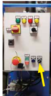
Start/Stop auxiliary pump for particle counter
