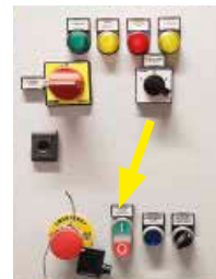
With electric indicator and particle counter Fig.11
