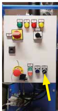
Start/Stop auxiliary pump for particle counter
