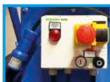
3-phase electrical panel
