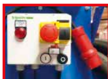
Single-phase electrical panel
